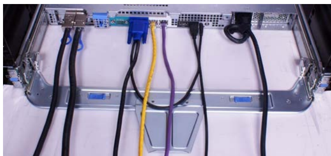
Figure 1. System with cables installed
